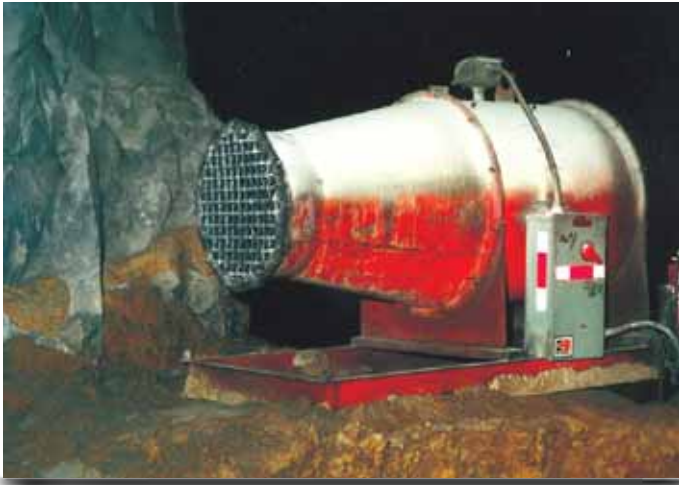
Figure 2: auxiliary Fan type used near face.
