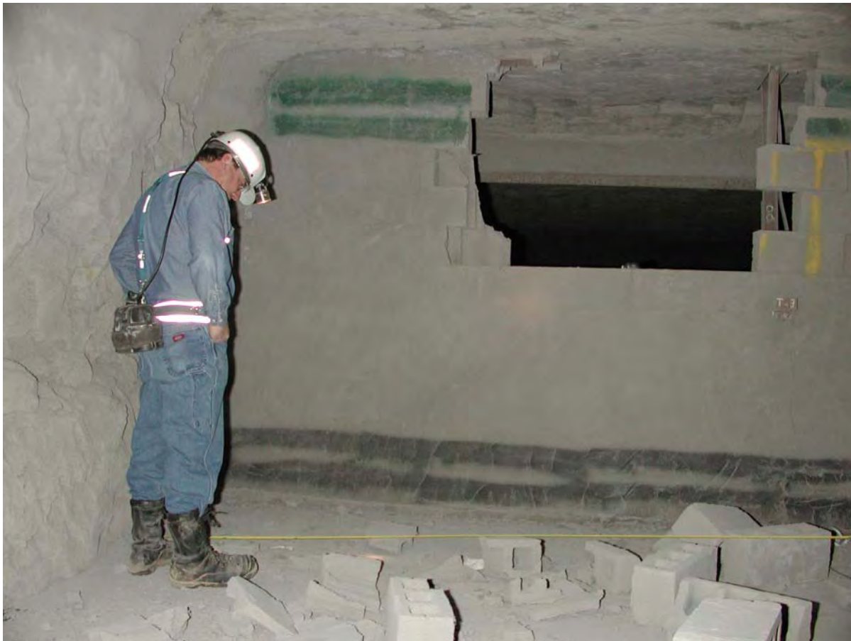
Figure 1. Ventilation stopping partially destroyed by explosion pressure
