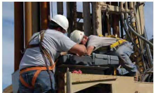
Figure 2. Installation of a uni-directional cab filtration and pressurization system. The uni-directional system delivers all of the filtered air into the enclosed cab at the roof and pulls all the recirculated air from the cab floor into the main filtering unit to be re-cleaned.
