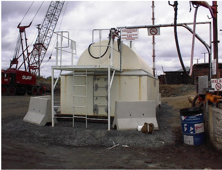
Figure 21 - Blended Fuel Storage on Surface
