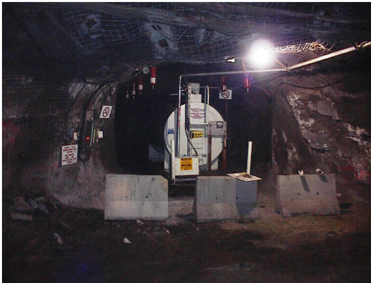
Figure 22 - Blended Fuel Storage at 1000 Level
