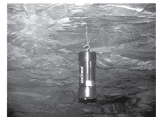
Radio Repeater Underground
