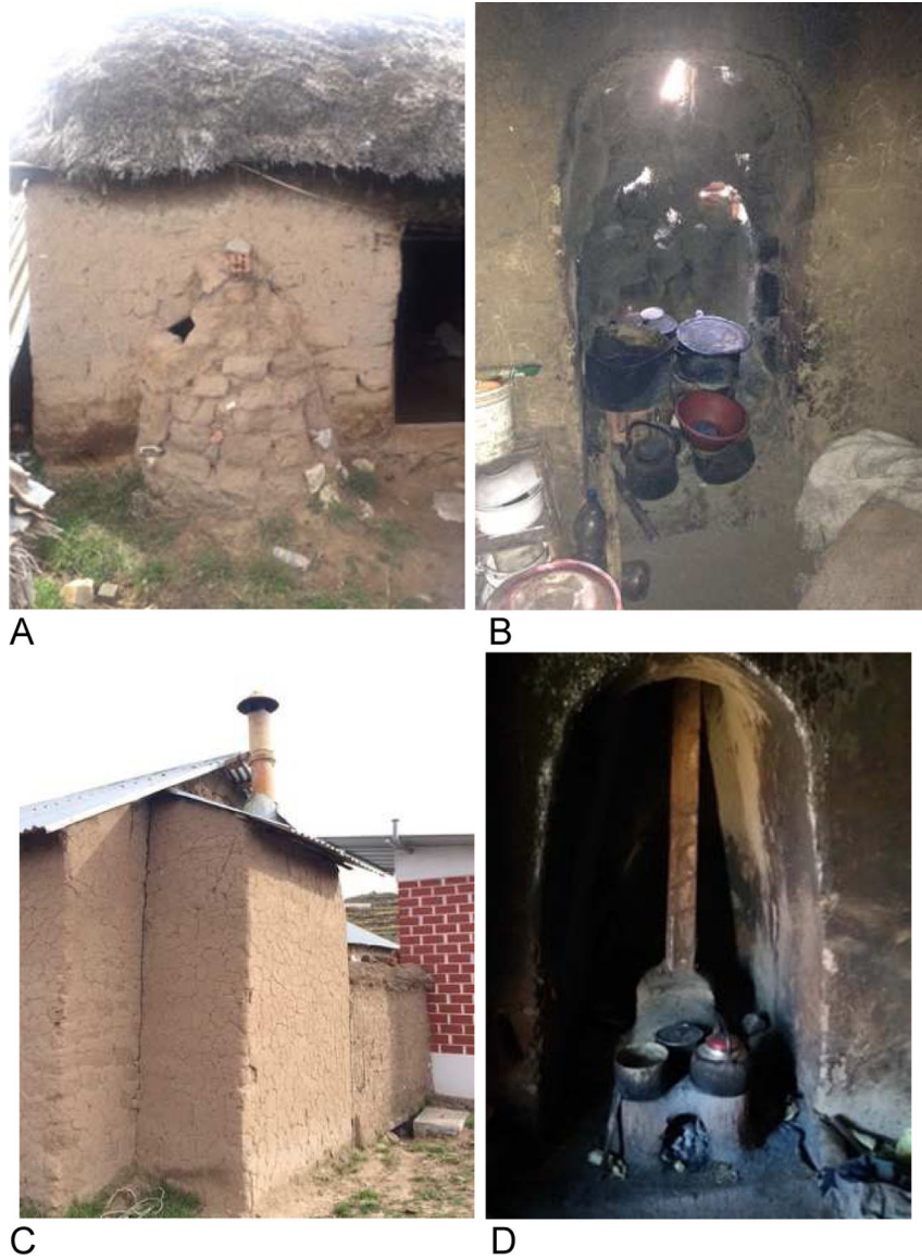
Figure 4. Examples of traditional stoves located in recessed areas in the kitchens of study participants (A, B) and chimneys used by study participants with traditional stoves (C, D).
