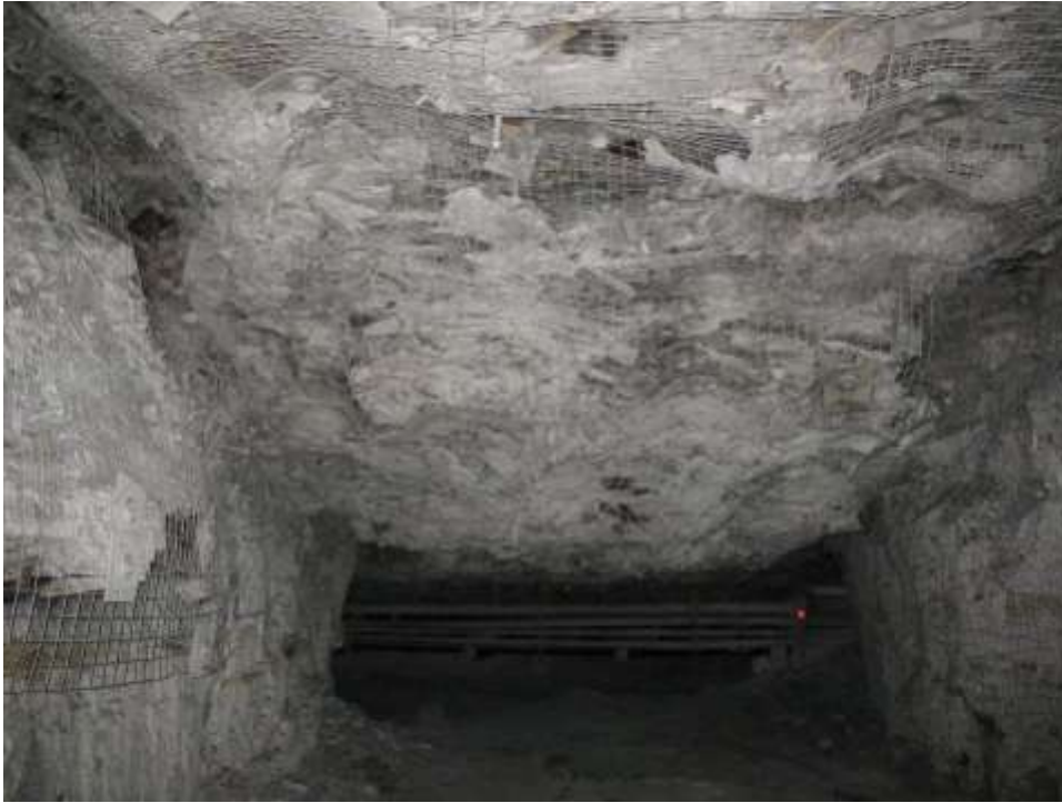
Figure 16: Heavily loaded roof screen preserves roof integrity.
