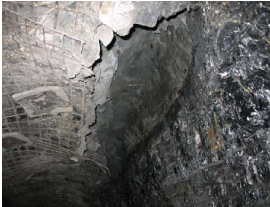
Figure 17: Exposed corners in wide entries can lead to guttering and eventually roof fall.
