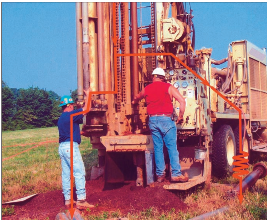
Figure 2. This photo shows possible electrical current paths to ground through a drill rig and a driller's helper during an overhead power line contact accident. This helper would probably be seriously injured or killed.
