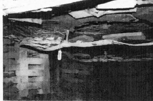
Figure 17. Rear abutment stress damage in L1 entry
