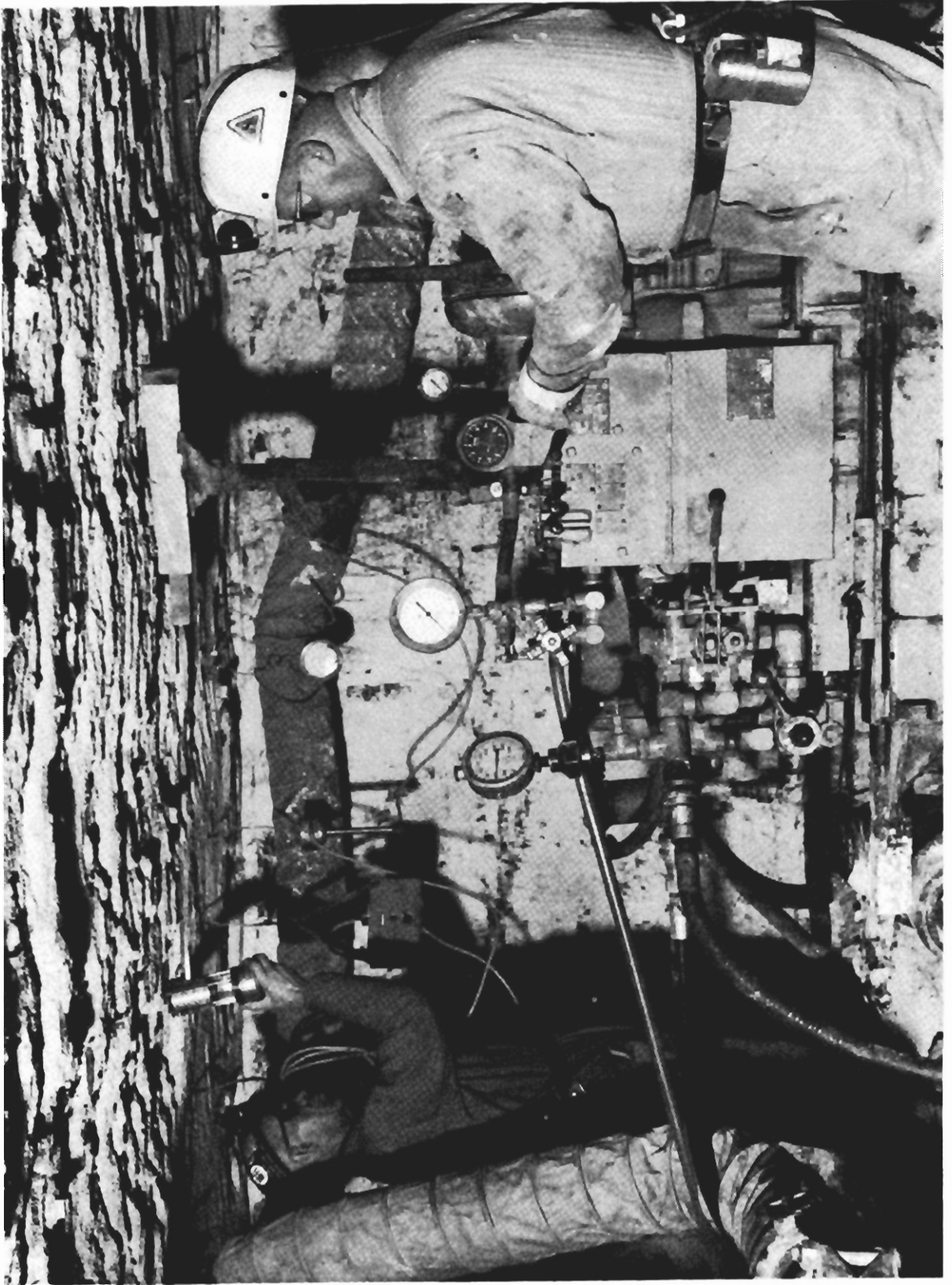
FIGURE 12. - Pressure gage and vent tubing.
