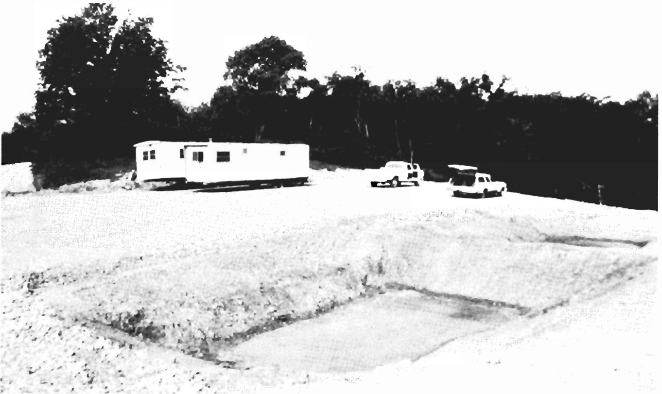
FIGURE 4. - Drilling location after site preparation. Mud pits in foreground. Photograph taken August 1978, view is northwest.
