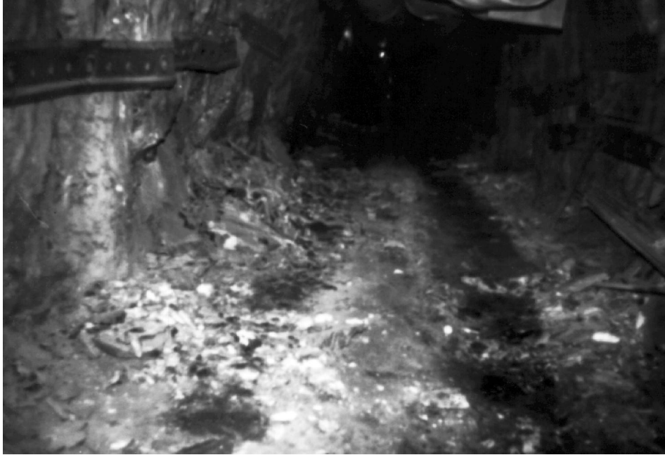
Sloughing on stope side of hanging wall drift. Shaft side remains intact. Note pronounced foliation.
