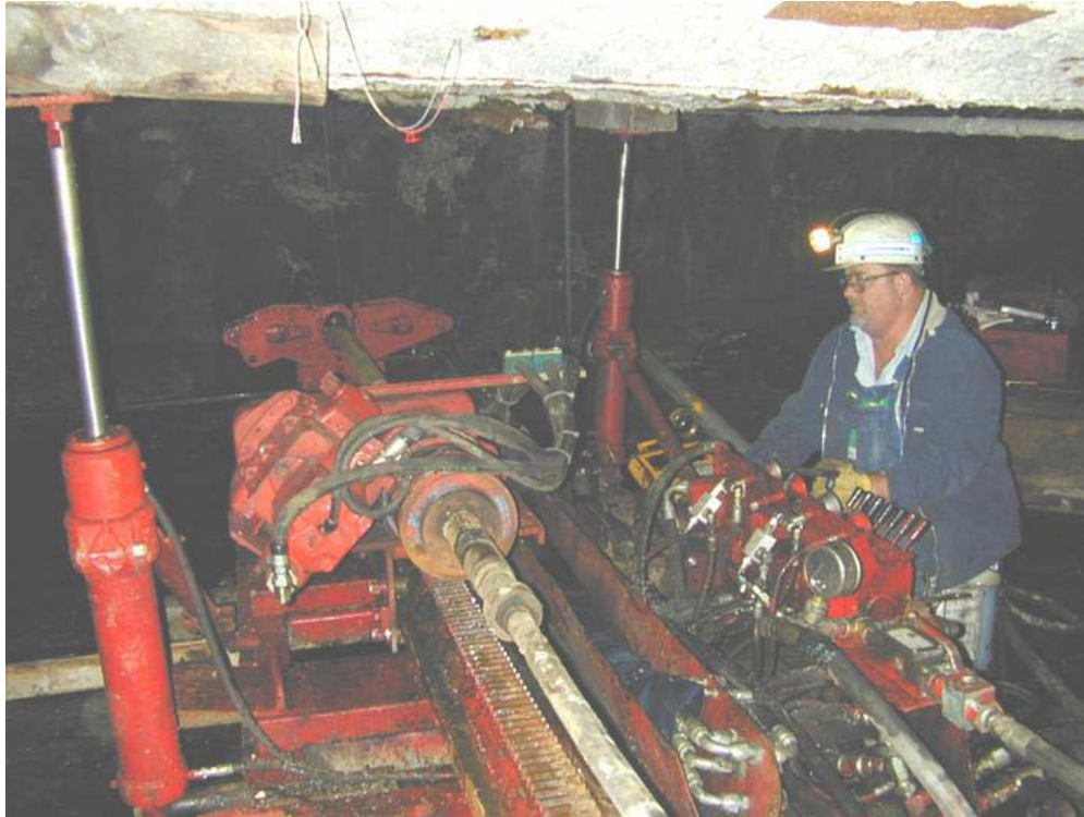
Figure 17. Photo of electrohydraulic drill rig that was used to drill the horizontal borehole.
