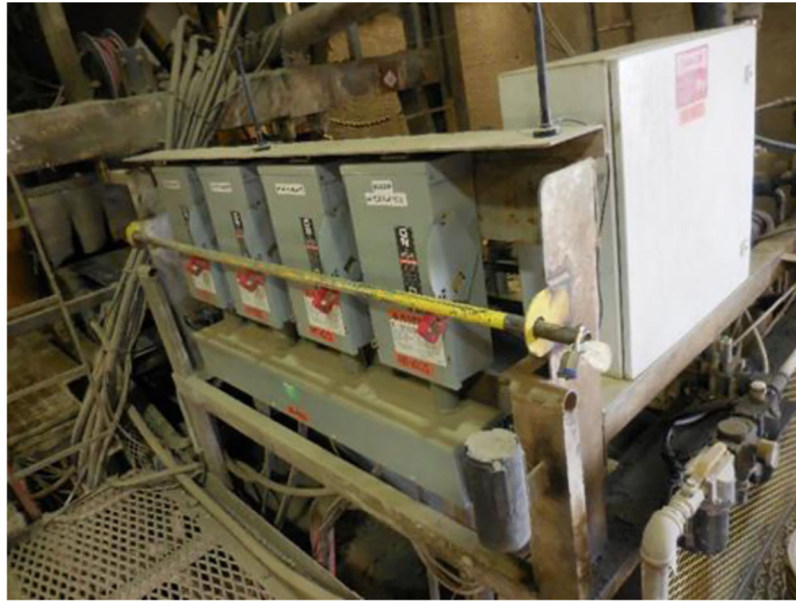
Fig. 2. Locked out disconnect panel
