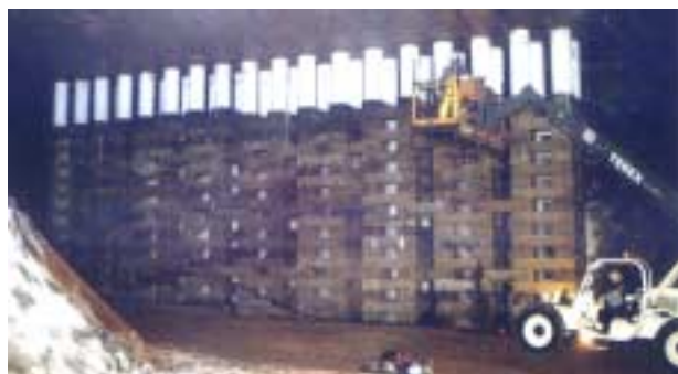
Figure 8. New crib wall C covering the crosscut in front of damaged crib wall.
