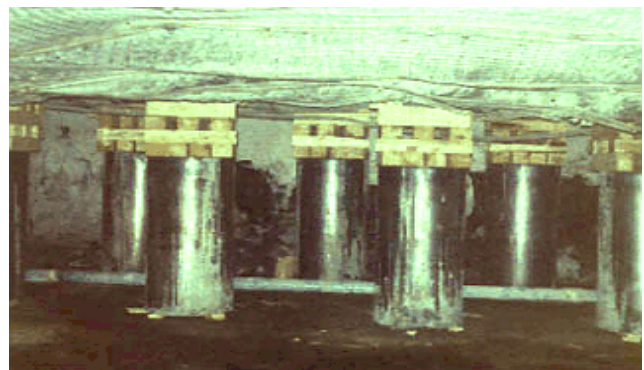
Figure 3. The Can support has replaced wood cribbing and is now the dominant secondary support used in western tailgates.
