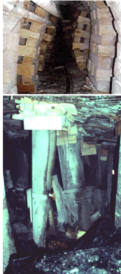
Figure 1. The compatibility of standing support with the loading conditions is essential for western longwall operations.
