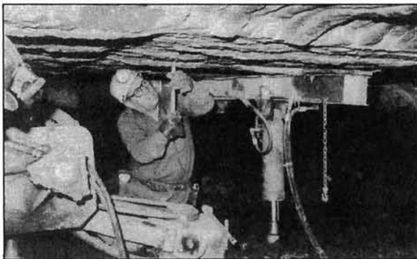
Figure 8.—Bolts installed in the mine roof help to prevent roof falls, thereby preventing fatalities and injuries to underground miners.
