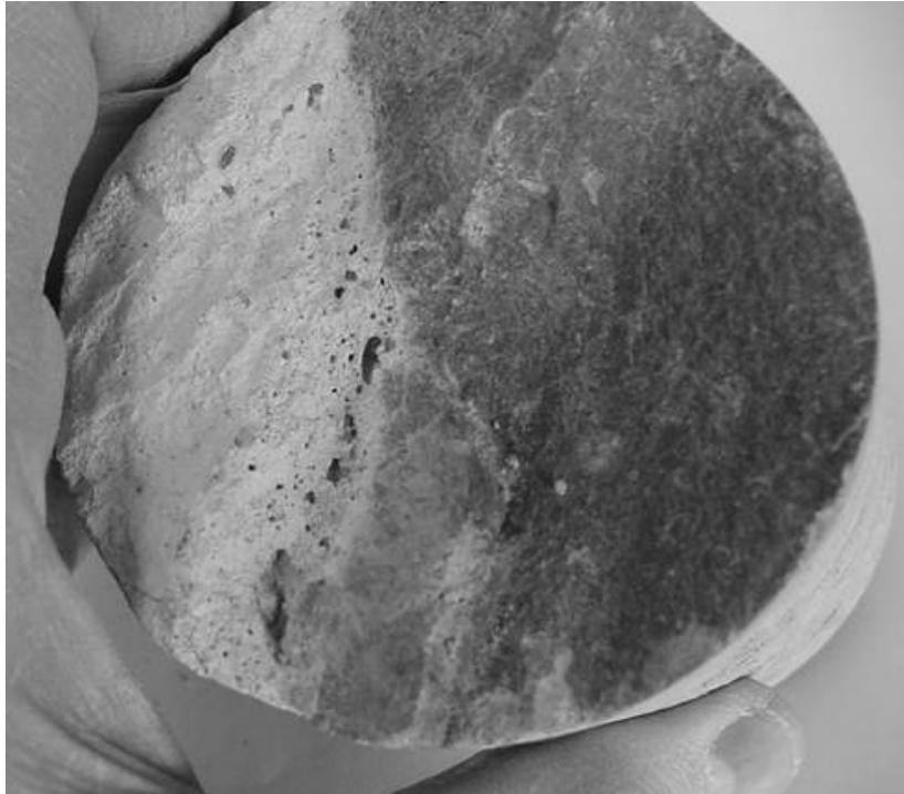
Figure 15 - Fine shotcrete coring with poor bonding at the rock/shotcrete interface due to air pockets and bubbles.
