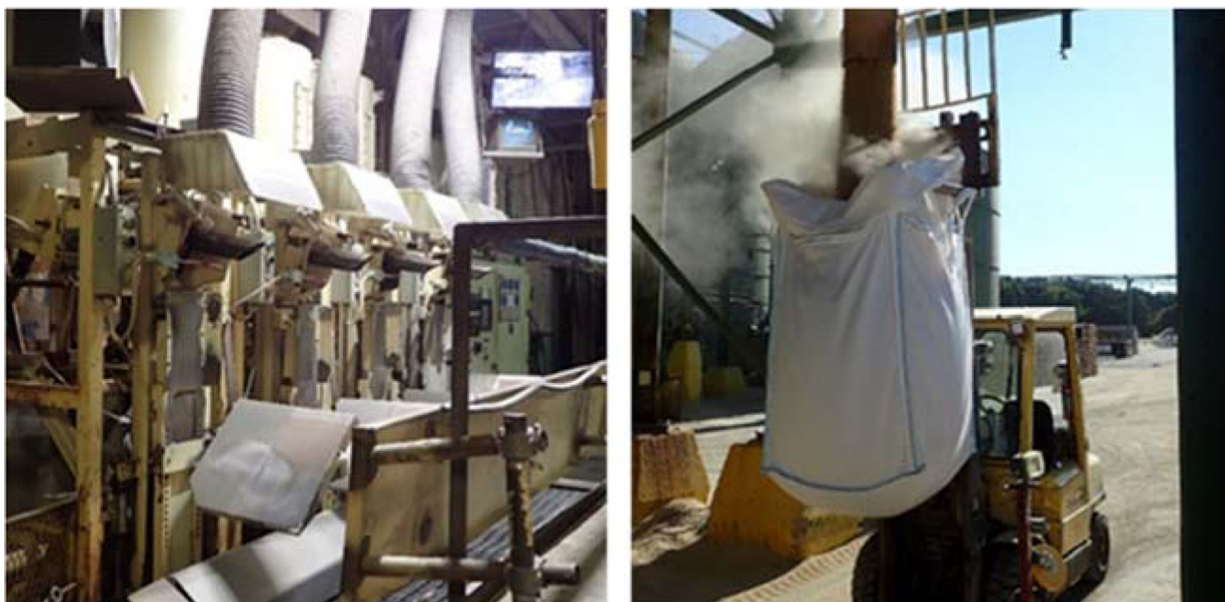
Fig. 8. Left: Manual bagging station with overhead LEV system. Right: Bulk bagging operation
