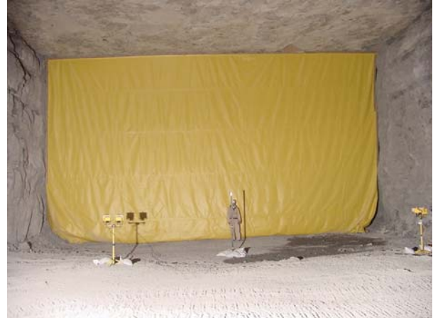
Figure 8. Tightly installed brattice stopping in a large-opening mine [16.8 m x 8.5 m (55 ft x 28 ft)]
