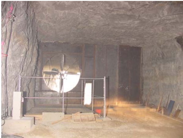
Figure 6. Large propeller fan mounted in bulkhead
