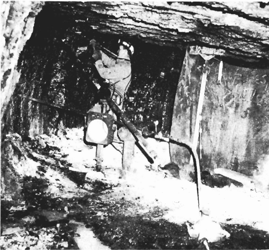
FIGURE 9. - Typical Arrangement of Infusion Equipment at Face; Sampling Air at Face-Sampling Point.
