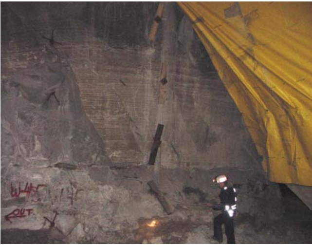
Figure 4. Typical common example of brattice being pulled from rib.
