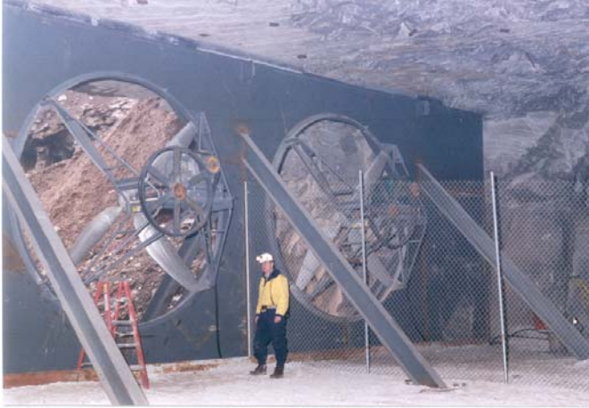
Figure 3. Two propeller fans installed for this study.
