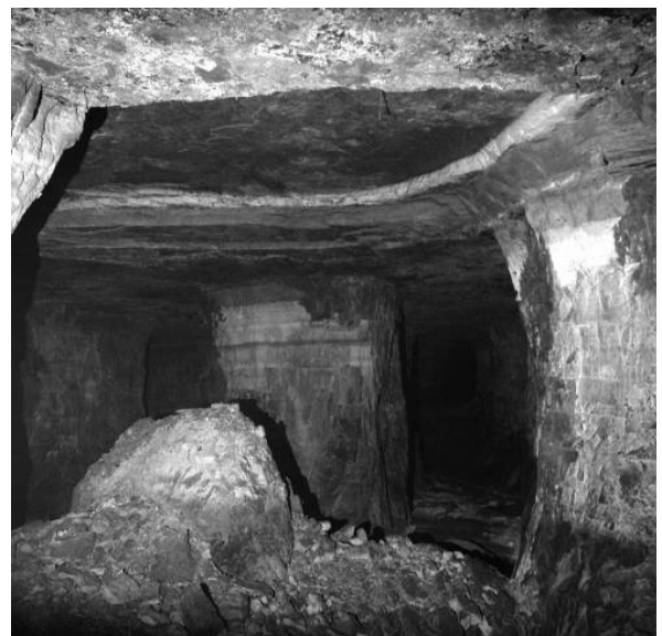
Figure 4. Stump of failed pillar at Mine B, showing roof failure at location of pillar and limited spalling of adjacent pillars (Case 8 in table 5).
