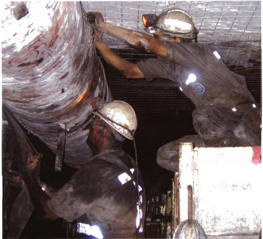
Handling vent tubes while at height increases falling risks.
