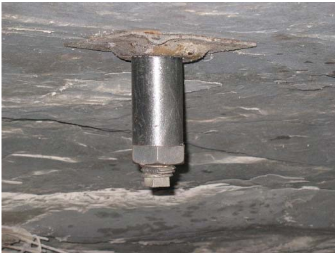
Figure 8. A "Ker-Thob" is used to re-establish plate contact with the roof and maintain roof bolt integrity.
