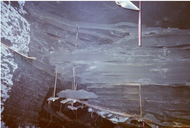
Figure 6. Roof fall in moisture-sensitive roof.
