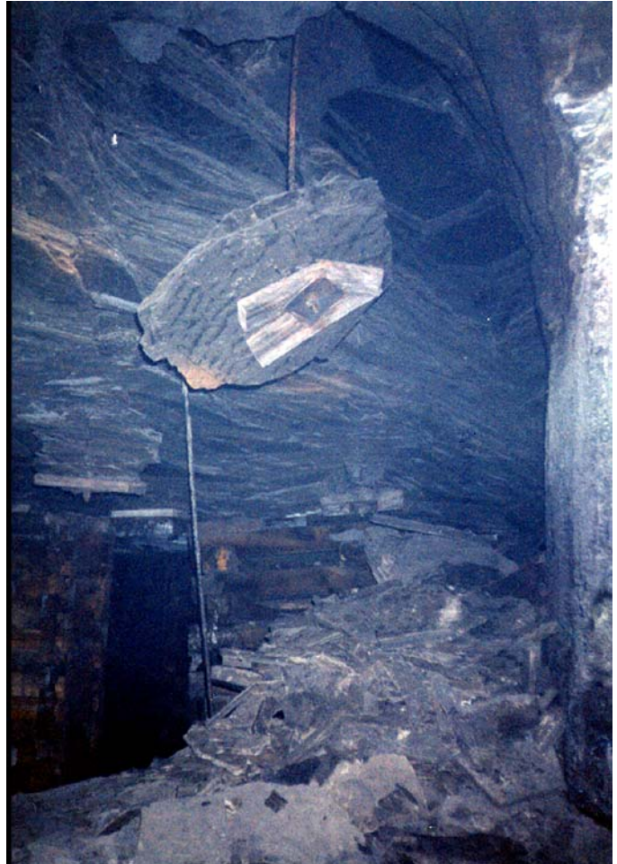
Figure 9. Severe guttering due to horizontal stress.
