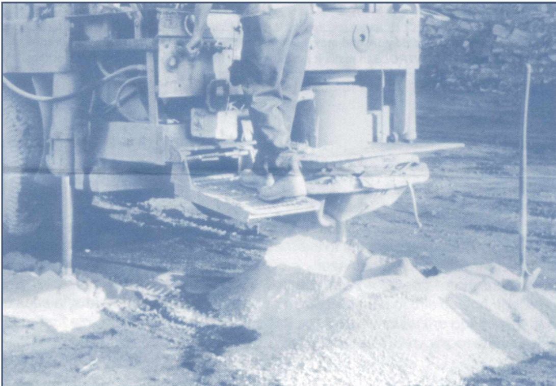
Figure 2. Drill operator at the control panel.
