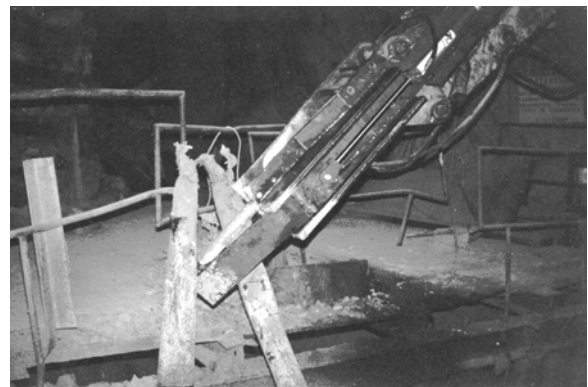
Figure 12.—Track-guided pincher arm picking up pipe debris from recessed grizzly
