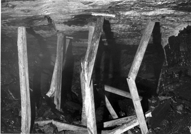
Figure 2 - Increasing the number of timber posts does not change their individual yield characteristics
