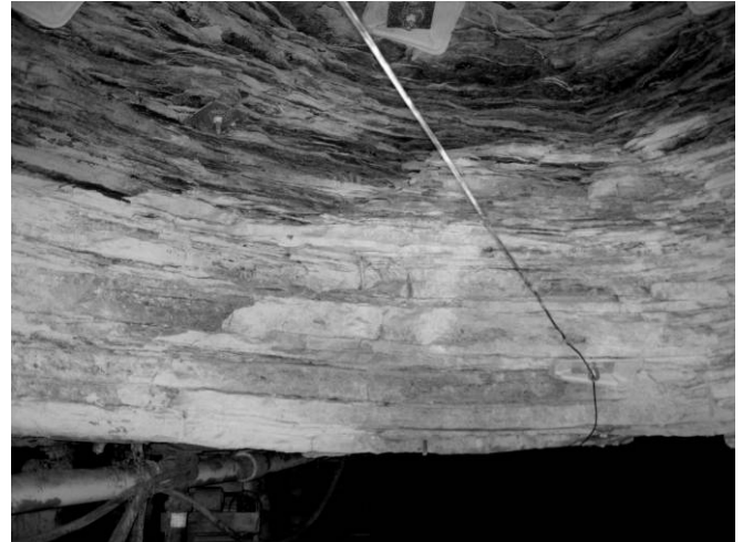
Figure 5. Section of roof adjacent to large roof fall.
