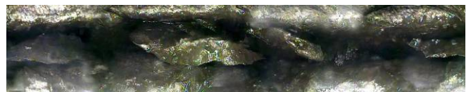
Figure 11. Void as observed from bore-scope video.
