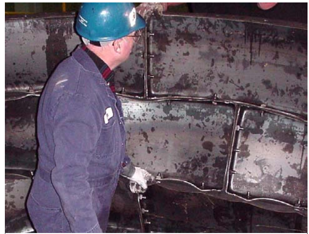
Figure 13. Vertical flange loading causes damage to the flange of the adjacent ring.
