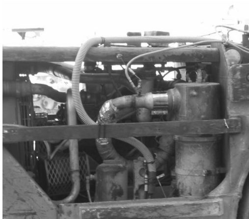
Figure 1. ArvinMeritor DPF system installation.
