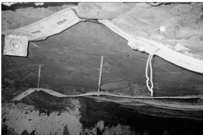
Figure 9. Water sensitive rock falls around bolts in an Illinois coal mine.
