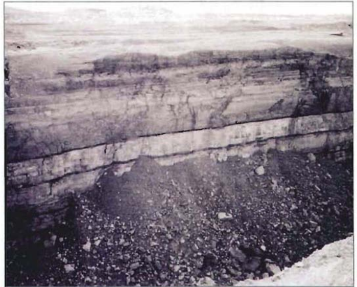
Figure 8-Site of massive web pillar collapse resulting in highwall slope failure. Photograph was taken from adjacent spoil pile. Highwall is about 150 ft high. A 110-ton coal haulage truck is buried in rockfall debris.
