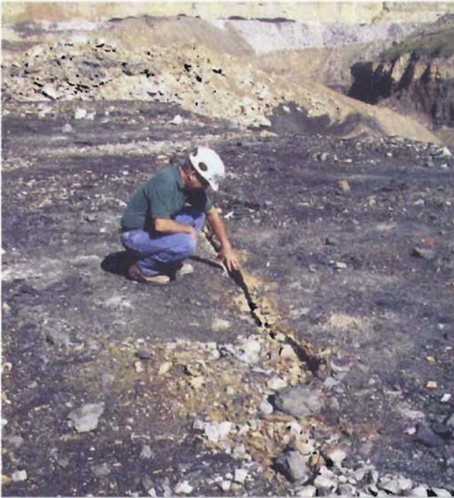
Figure 3-Crack in bench above highwall mining operation.
