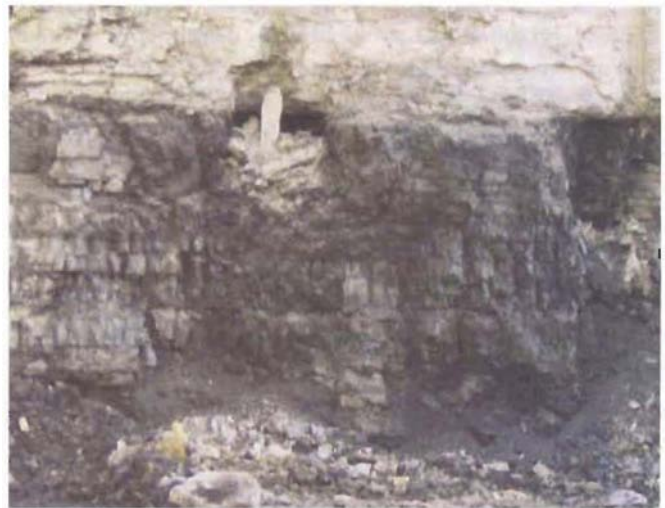
Figure 7- Old underground works daylighting in highwall can pose ground control hazards.
