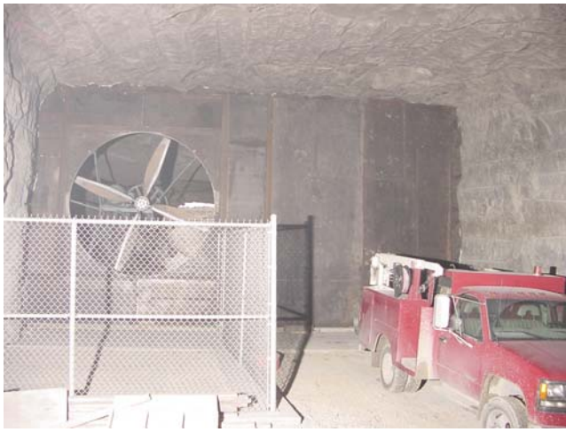
Figure 16. 3.66 m (12 ft) propeller fan mounded in a steel bulkhead.
