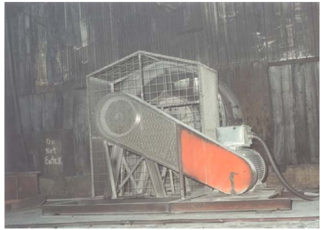
Figure 15. 2.44 m (8 ft) vane-axial main mine fan mounted in a sheet metal bulkhead.
