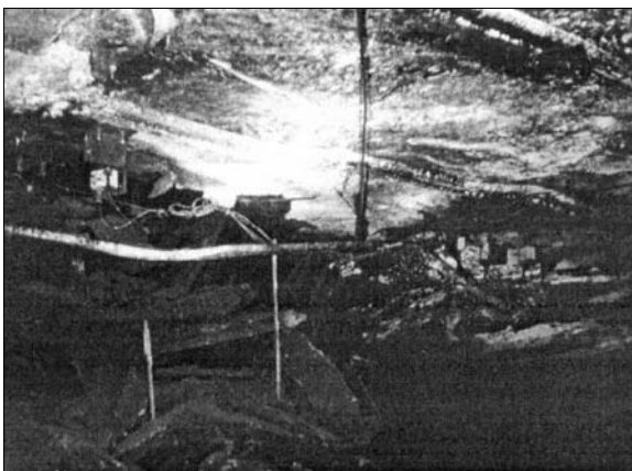
Figure 4. Photograph showing fully grouted bolts pulled from their holes in a roof fall.
