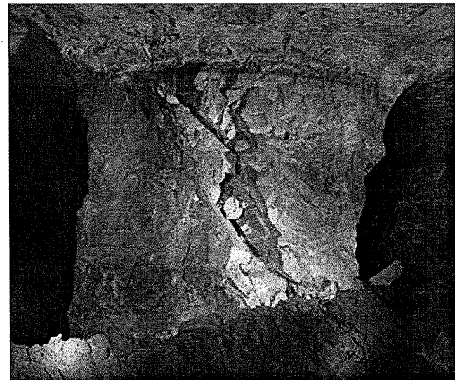
Figure 10 — Partially benched pillar that failed along two prominent discontinuities dipping at approximately 60°.
