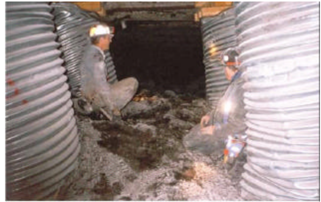
Figure 2. A longwall tailgate supported with 3C supports subjected to considerable convergence before useful support capacity is realized.
