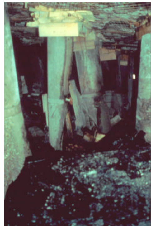
Figure 4. Failure of stiff concrete supports in a displacement-controlled environment.
