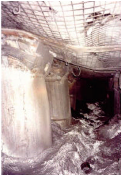
Figure 1. Large roof deformations resulting from a soft crib system.
