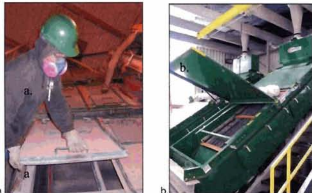
Figure 4. Old screen cover being removed from housing (a) and new screen cover retrofitted with gas struts (b).
