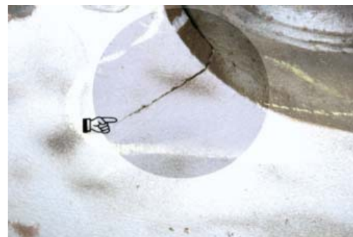
Figure 9 Failure of base rib side plate where fabrication process left large flaws
