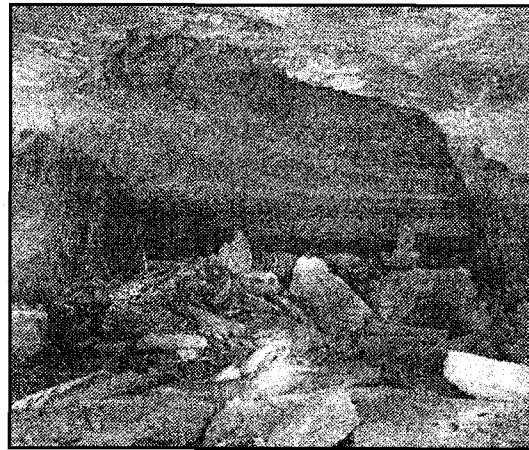
Figure 4. - If the roof is not reinforced properly with rock bolts, the beams can progressively fail higher into the roof until a stable roof beam is encountered. Here the roof fall has assumed an elliptical shape.
