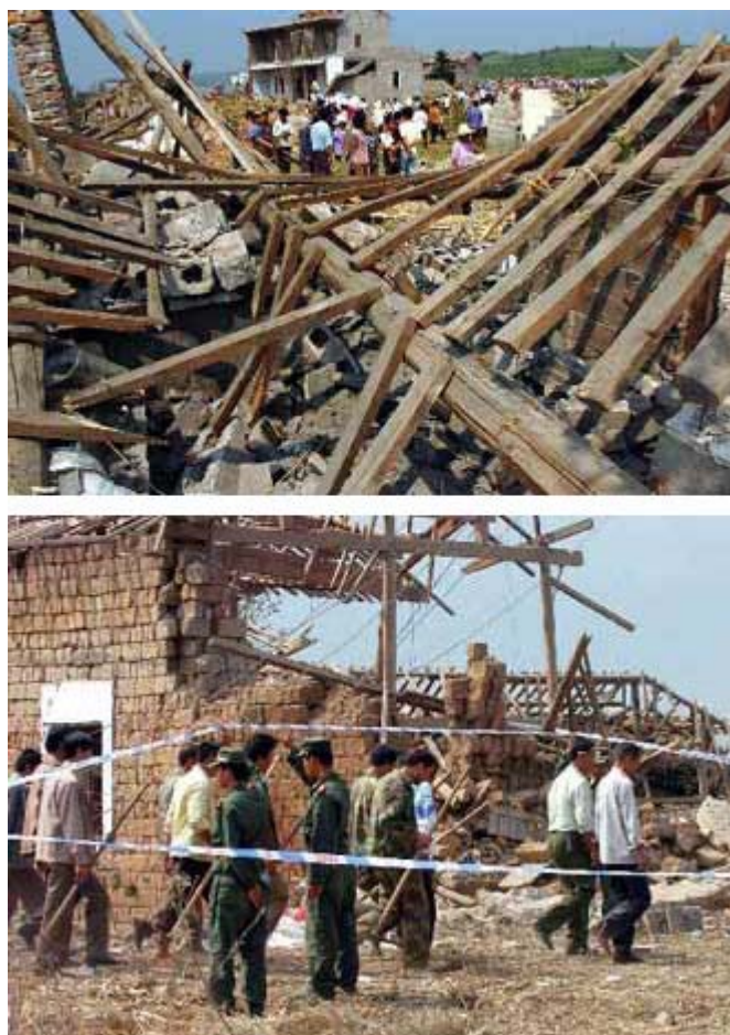
Figure 5. Damage caused by the 2005 explosion of an 18-MT (19.5-t) truckload of AN in Zhenganzhai, China.
