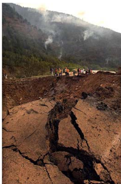
Crater and damaged roadway
