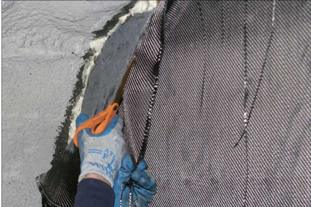
Figure 22.—Cutting the woven CFRP base wrap to match the contour of the mine rib and roof.
