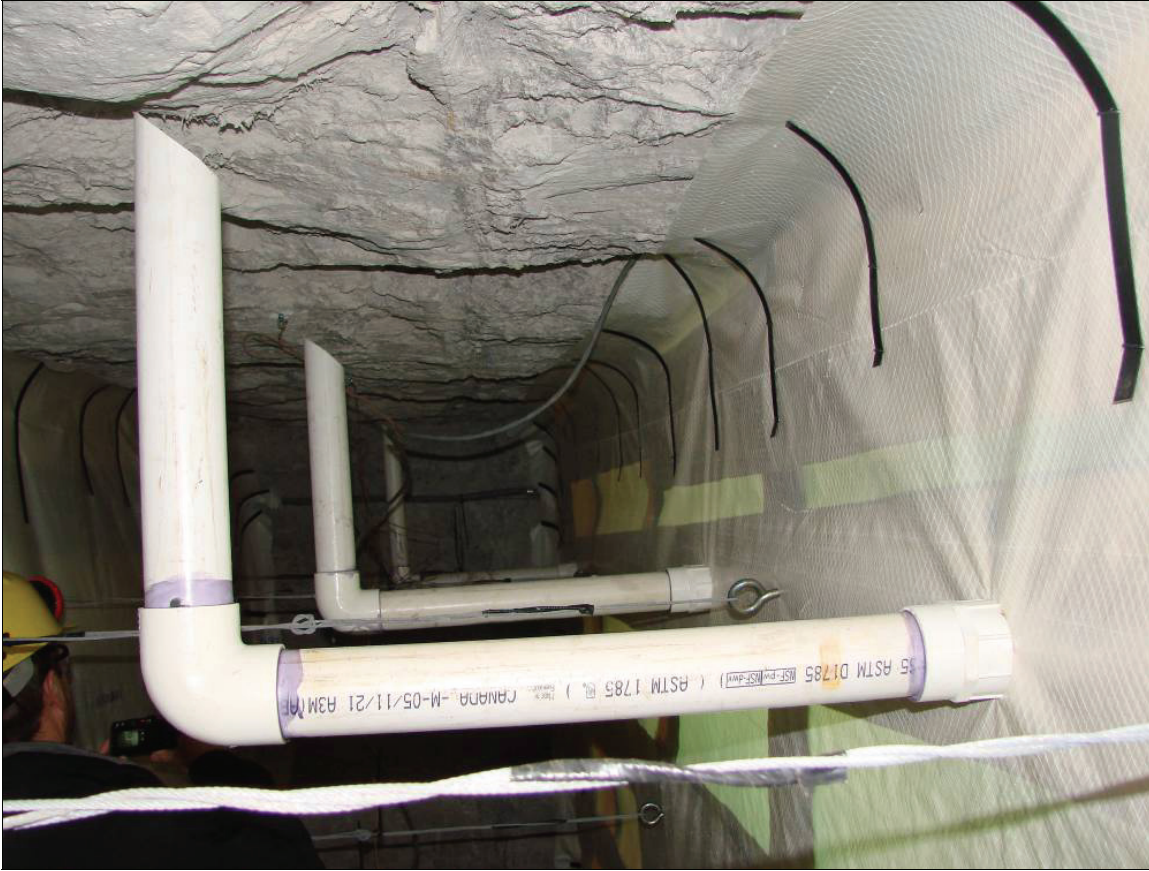
Figure 7.—View between the two form walls showing the injection and bleeder pipes, the flexible metal straps holding the overlapped brattice tight to the strata, and the steel cable ties between the inby and outby form wall posts.
