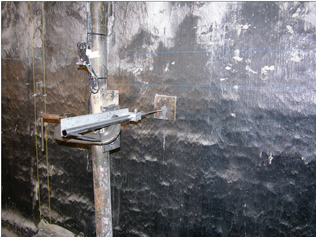
Figure 4.—LVDT mounted behind seal to measure movement of the seal during an explosion. The vertical yellow wires to the left of the sensor post and the horizontal blue wires above the LVDT anchoring plate on the seal are the breakwires.
