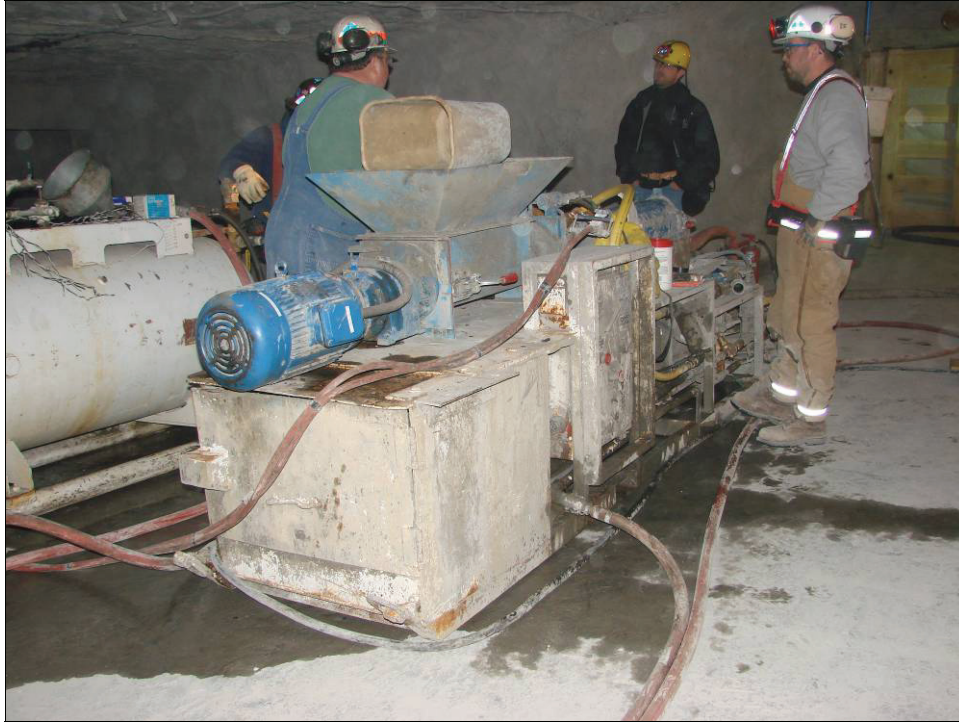
Figure 8.—Electric-powered screw auger ( center of photo ) for the cement feed and the heated water and foam tank ( left side of photo ).
