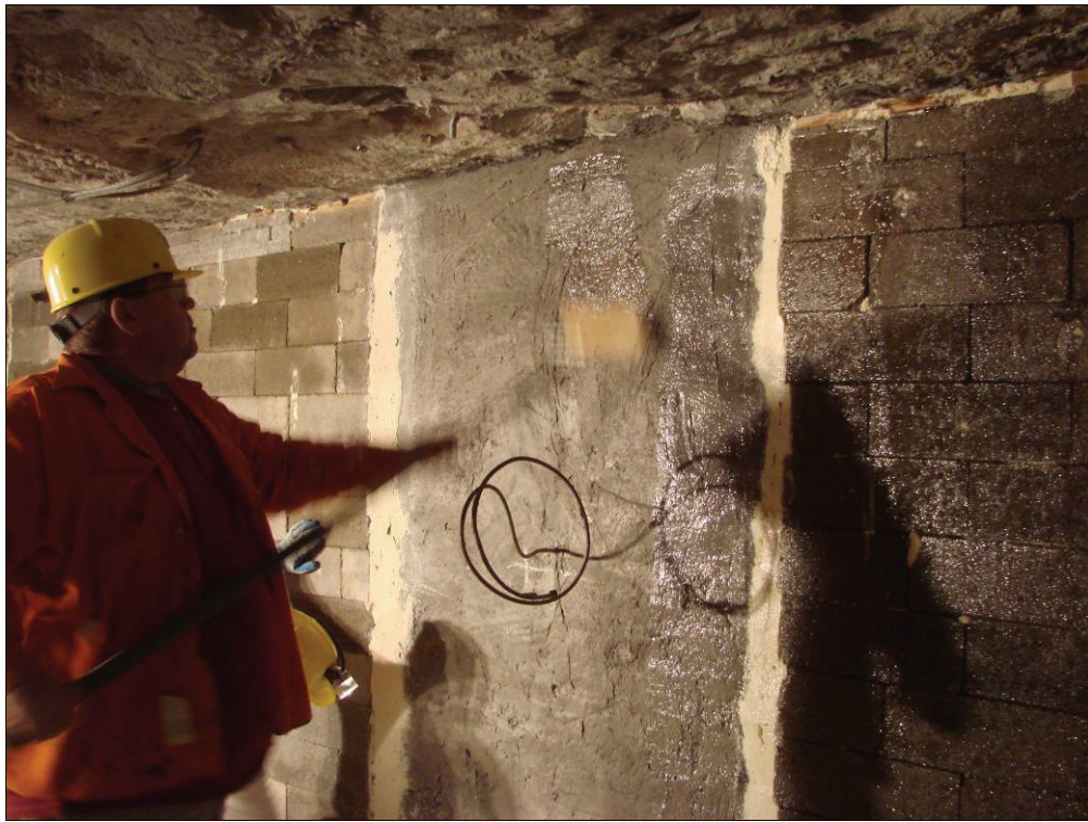
Figure 27.—Applying the primer resin with a paint roller to the concrete block and pilaster.
