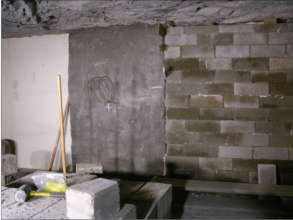
Figure 26.—Completed block wall to the right of the pilaster and the installed rigid urethane board to the left.
