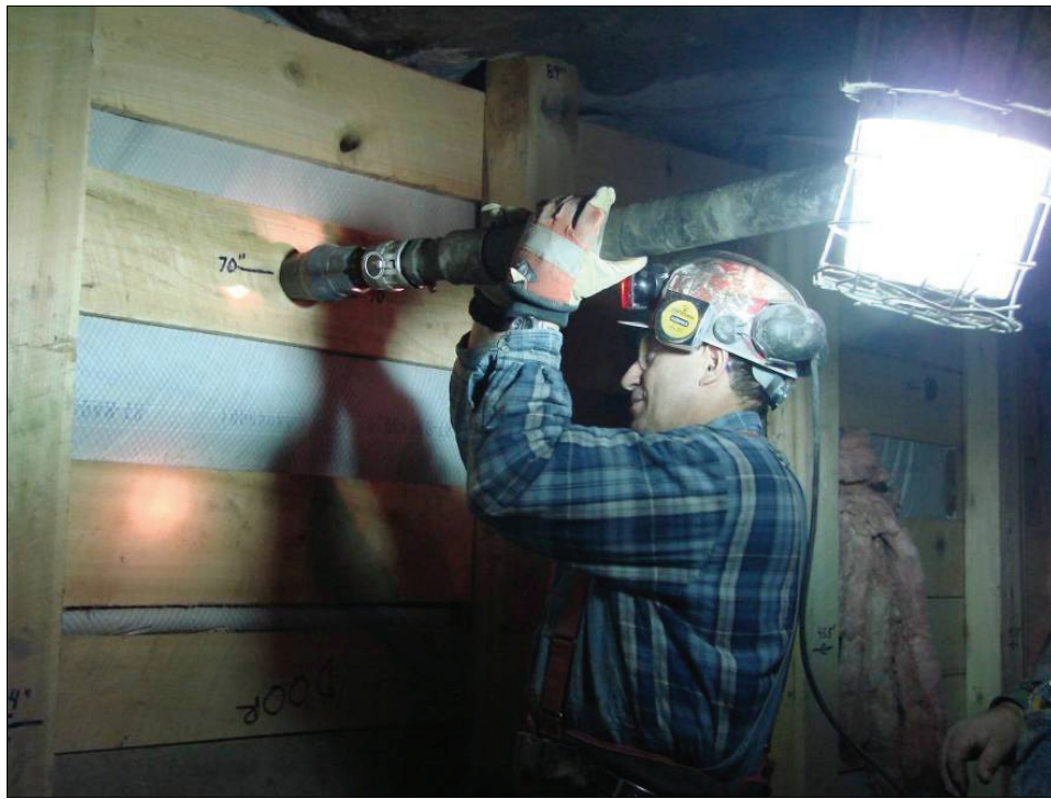
Figure 11.—Connection of the slurry injection hose for filling the top third of the seal.
