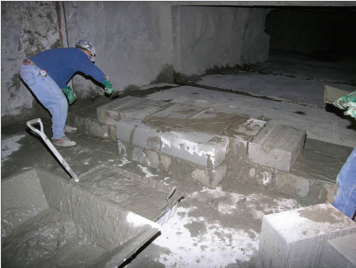
Figure 13.—Full wet-bed construction on all horizontal and vertical block joints. The vertical block joints are staggered.
