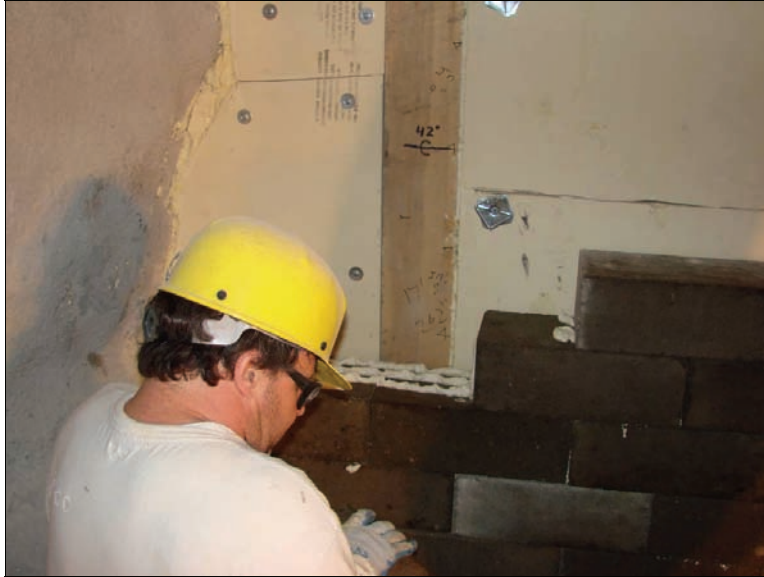
Figure 19.—Construction of the solid-concrete-block wall. A one-component foam adhesive was used on all of the block joints.
