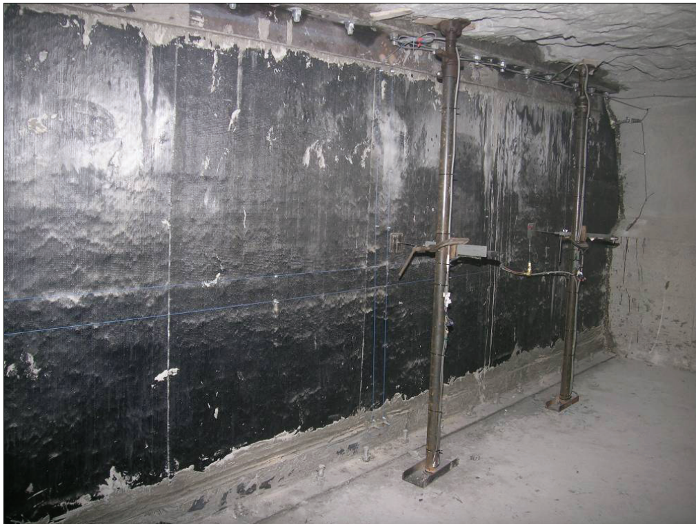
Figure 23.—Completed CFRP reinforcement retrofit to the C-320 pumpable cementitious foam seal, and the LVDT displacement sensors mounted to posts and attached to seal.
