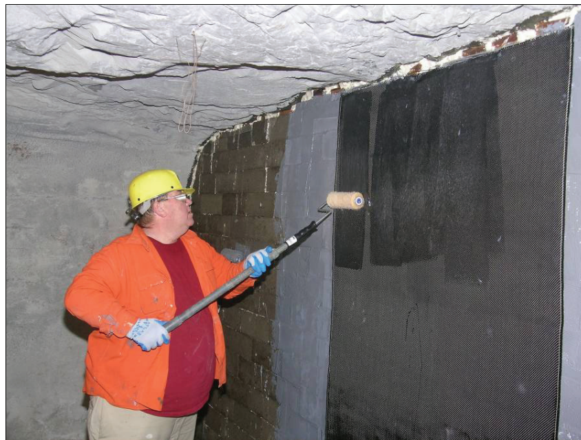
Figure 21.—Applying the resin saturant coat over the CFRP base wrap. The light gray undercoating on the concrete block is the resin tack.
