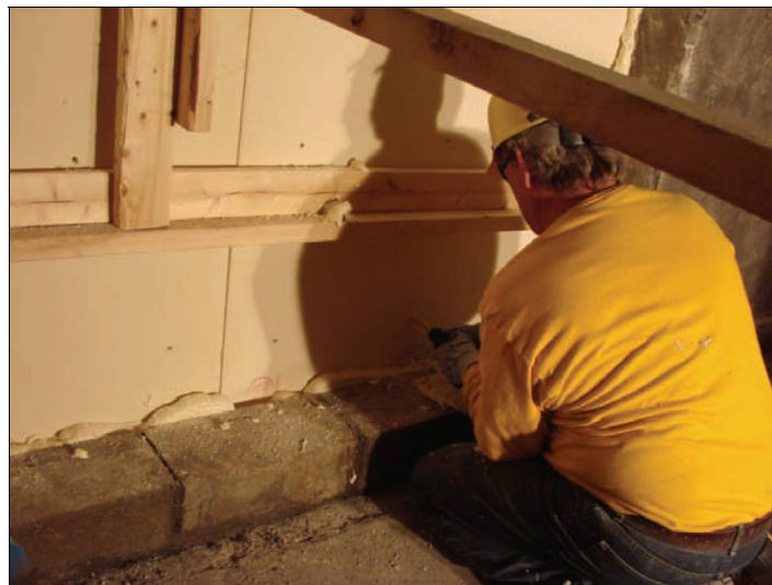
Figure 25.—Injection of the two-component polyurethane foam at the perimeter and behind the rigid urethane board.
