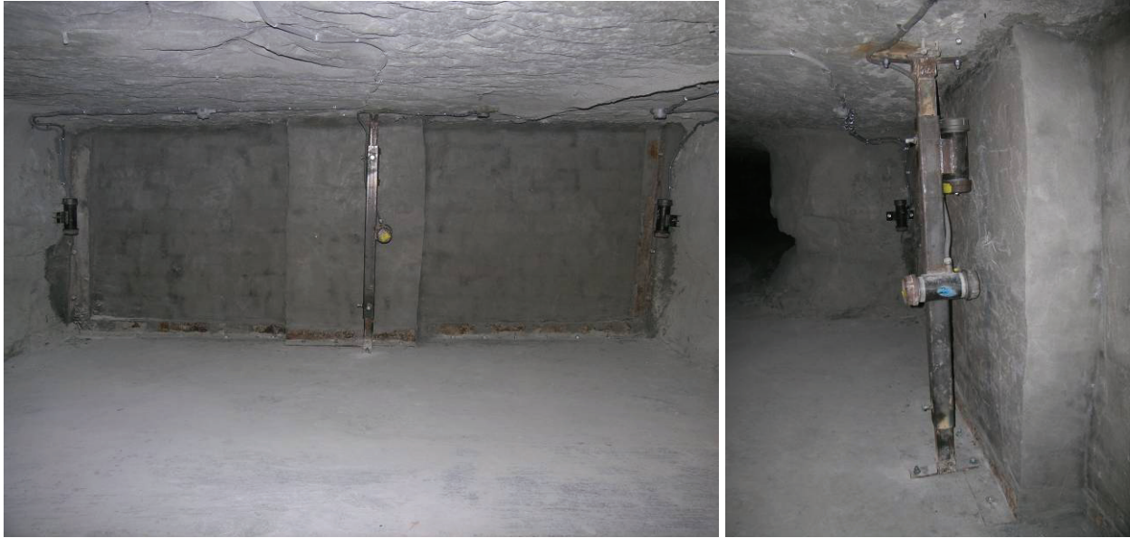
Figure 3.—Front view ( left ) and side view ( right ) of housings and mounts for the pressure transducers on the explosion (or C-drift) side of the low-density block seal in crosscut 3.
