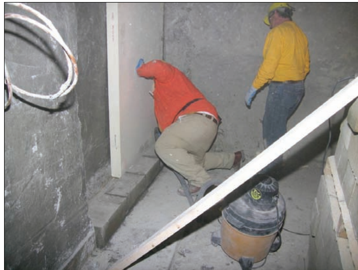
Figure 24.—Positioning the rigid urethane board between the first course of concrete block and the seal.
