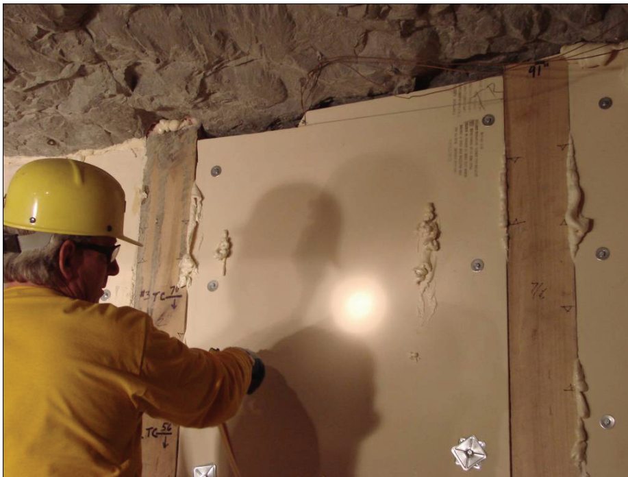
Figure 18.—Injection of the two-component foam behind the rigid urethane board that was secured between the form wall posts with lag screws.
