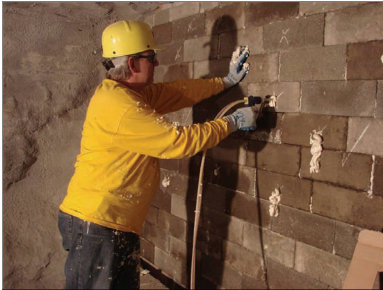
Figure 20.—Injection of the two-component foam through the block to fill the 1-in gap between the seal and concrete block wall.
