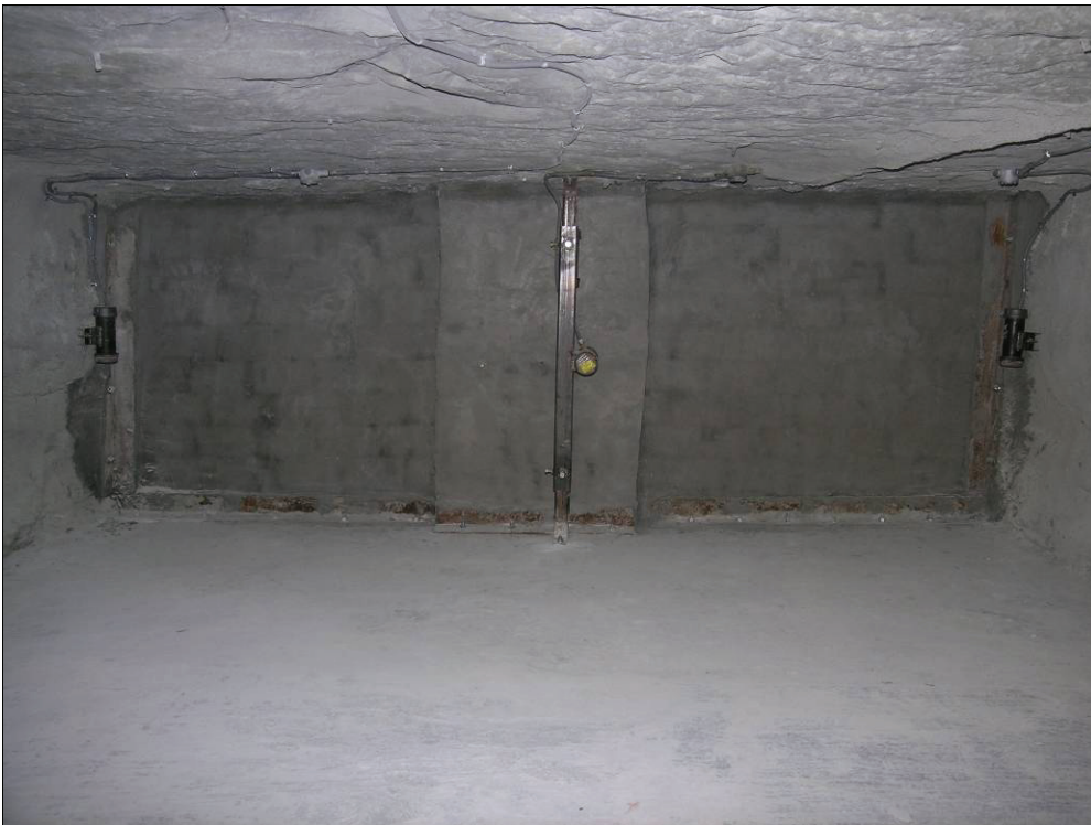
Figure 17.—Completed 24-in-thick, low-density block seal as seen from the C-drift (explosion) side.
