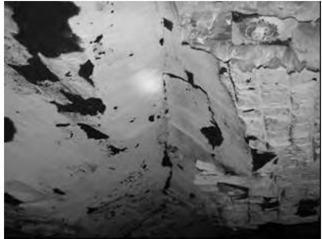
Figure 1.—Roof fall initiated by unfavorably oriented slip planes.
