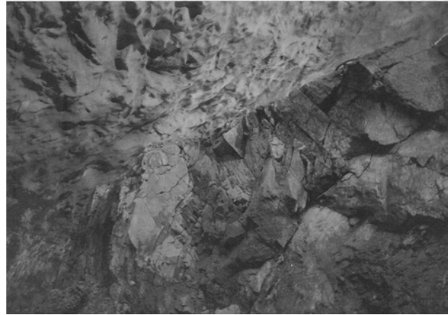
Figure 6.—Example of a well-jointed rock mass with most typically J_n = 9 (three sets of joints) and J_r = 2 , seen in the Gjøvik Olympic cavern of 62-m span. Note the deep overbreak in the 25-m-high arch and the use of B + S(fr) permanent support [Barton et al. 1994].
