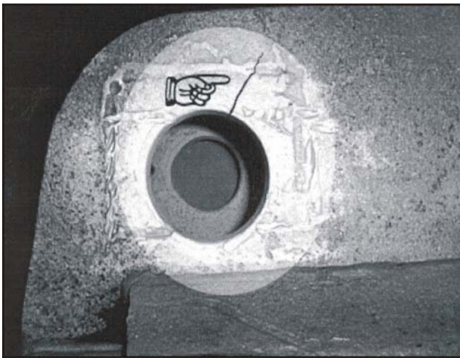
Figure 15.—Failure in base lemniscate link clevis.
