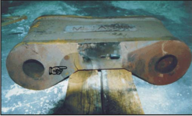
Figure 13.—Failure of bottom lemniscate link.
