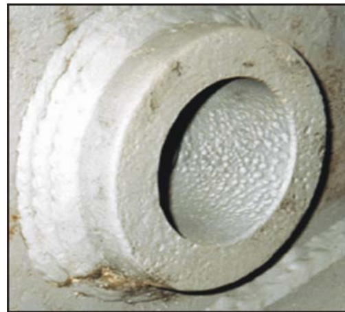
Figure 8.—Corrosion of a lemniscate link clevis.
