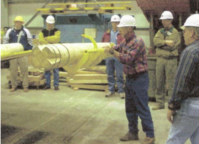
Figure 17.—Apparatus used for setting timber posts. (Photo courtesy of Strata Products USA).
