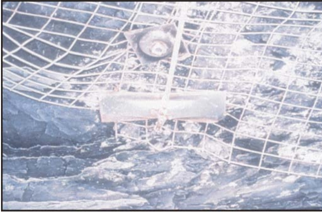
Figure 27.—Roof damage from horizontal stress around cable truss in headgate just outby the face.
