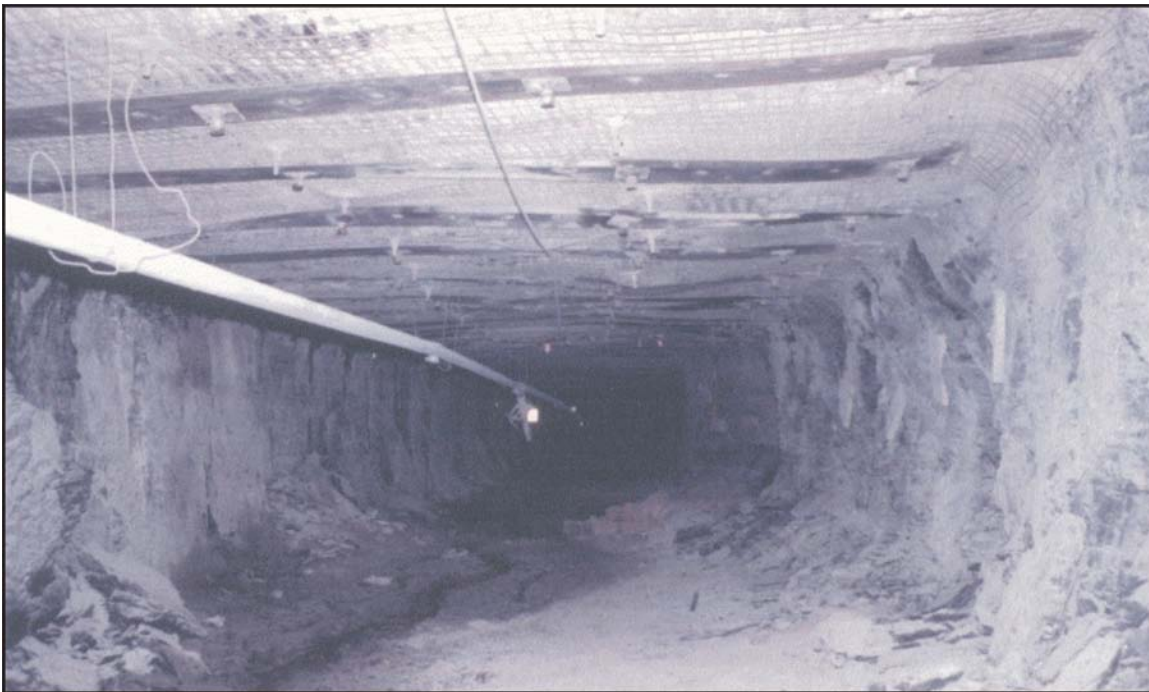
Figure 8.—Surface control in the form of a "Monster Mat" installed with cable bolts.
