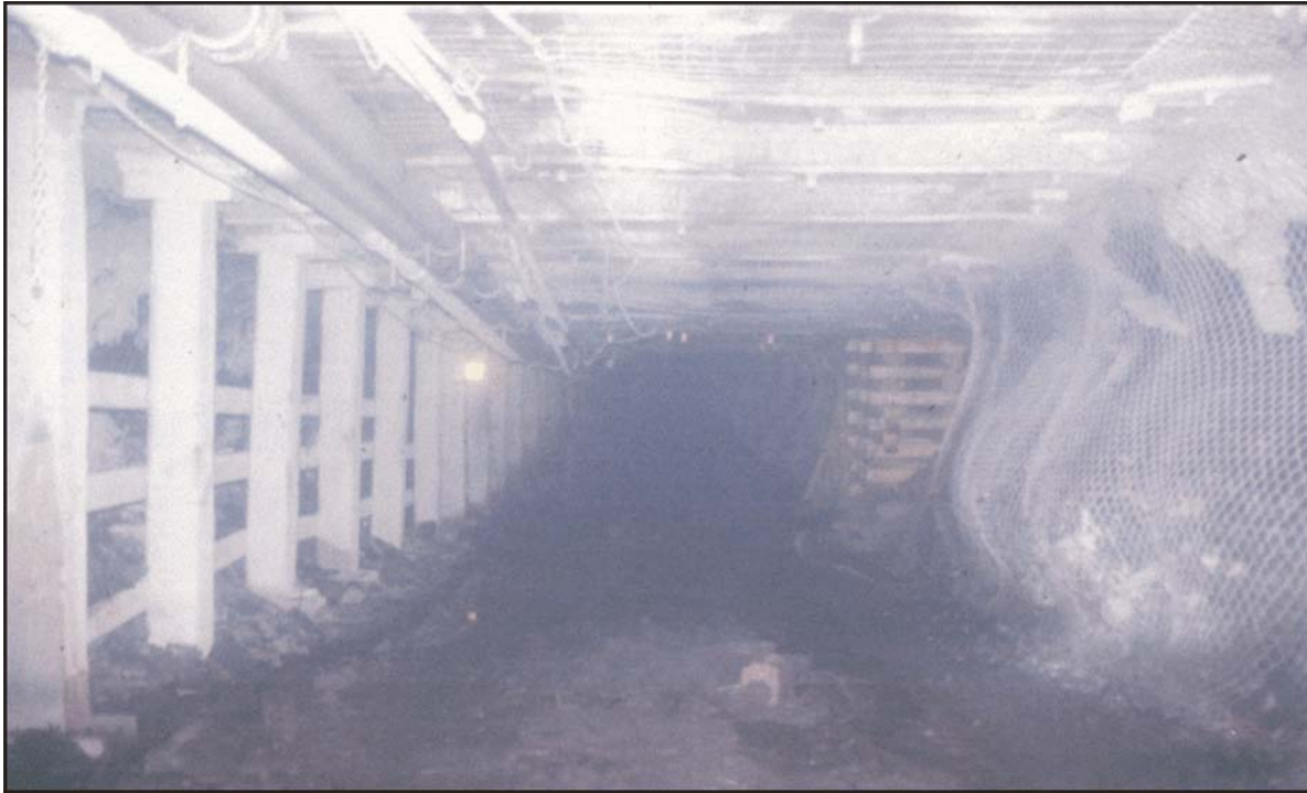
Figure 20.—Two entry yield pillar tailgate showing the abutment zone outby the face, supported with cable bolts
