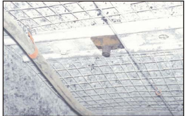
Figure 3.—Cable bolt system installed in a tailgate.
