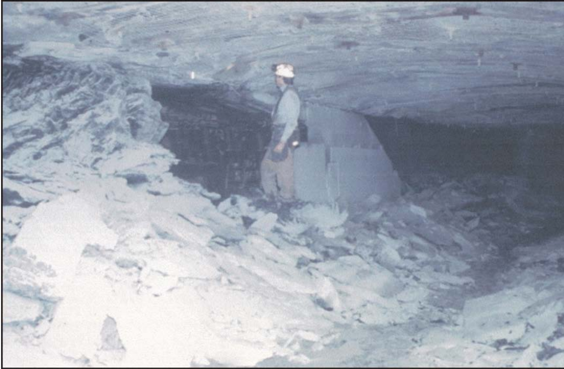
Figure 15.—Tailgate shield zone supported by cable bolts.
