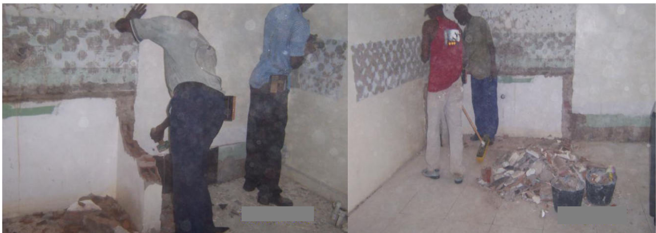
Figure 3. Photo of workers from Crew 1 breaking up masonry structure and clean-up demolition debris before worker training (Photographer: C.M.).
