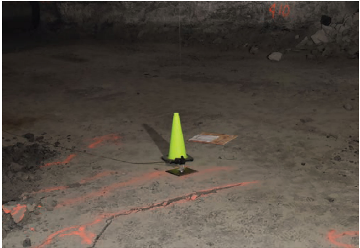
Figure 4 - Extensometer #3 located near a previously observed floor crack.
