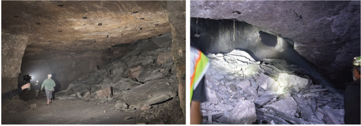
Figure 2 - Roof collapse area.
