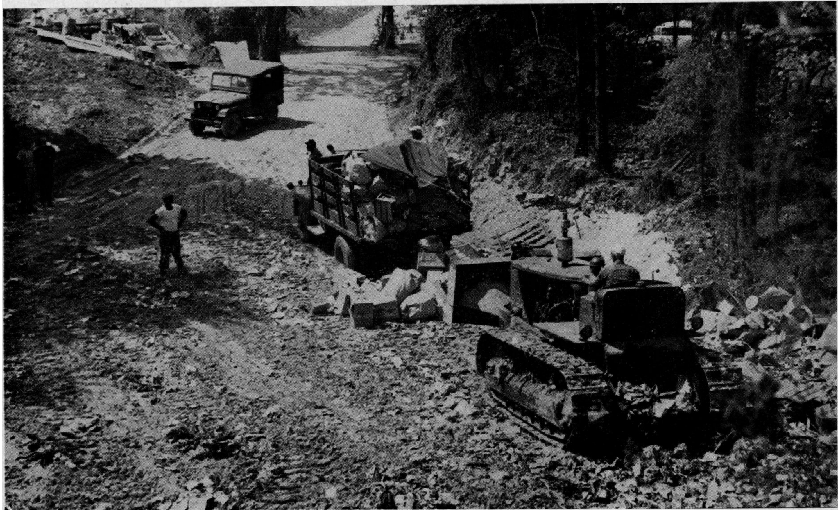
A stake-truck is unloaded at the site of the sanitary landfill in Pennsylvania. A front-end loader pulls at the front end of the tarpaulin, rolling out refuse.
